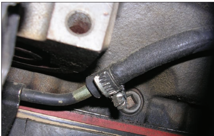
Since this hose is so hard to see, it often gets overlooked while troubleshooting a no-start situation.
