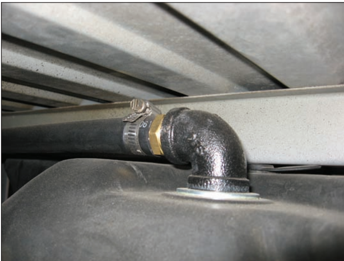
This shows the main-tank pickup tube in place with the tank installed. It is in the perfect position with no clearance issues, and connects to the Jabsco pump with a short run of hose that does not come into contact with any part of the truck bed or tank.
