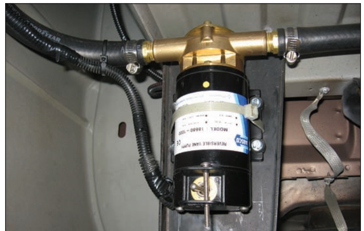
The Jabsco diesel pump I chose is typical of the type of pump used to transfer fuel to your main tank in many of the manufactured systems. This one differs in that it is reversible at the same flow-rate. The hose to the right connects to the fabricated pickup tube in the main tank. The center-off switch is used to reverse polarity to the motor. I installed the screw to restrict the switch to only one direction or off, because I am using a remote-mount switch to control the pump and want to maintain direction of fuel flow consistent with switch position. In use this pump-mounted switch has a rubber boot covering it.
